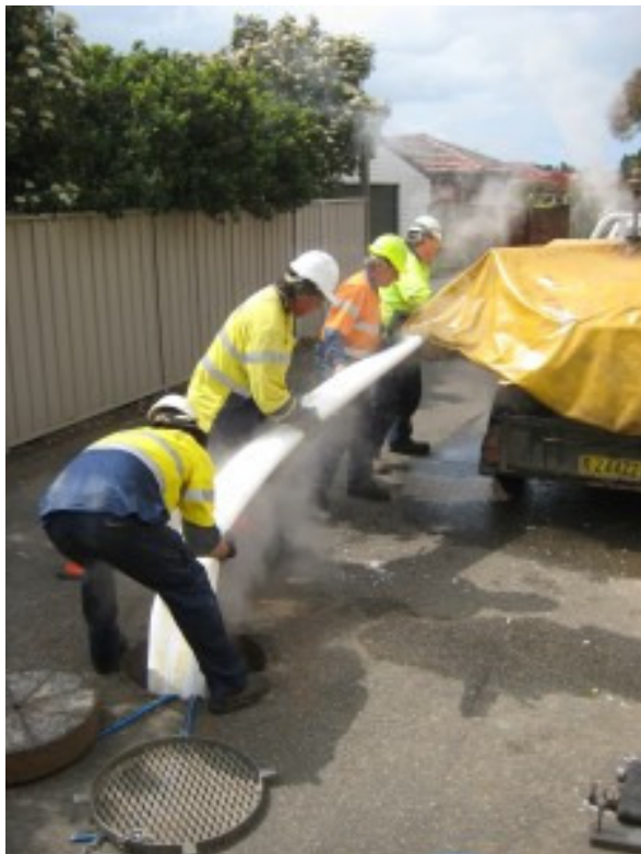
Figure 7: Fold and Form PVC pipe during installation (Photo courtesy of Kembla Watertech)
